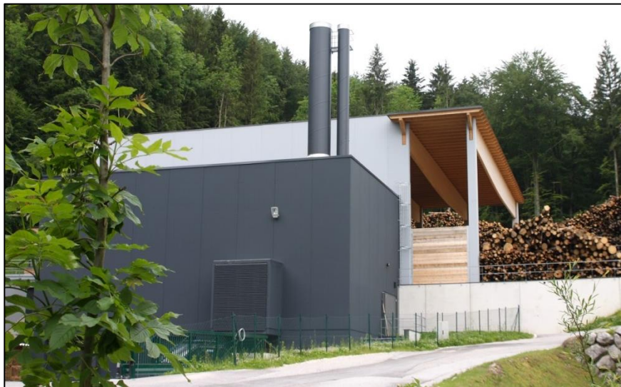
Heating plant in Fuschl am See.
